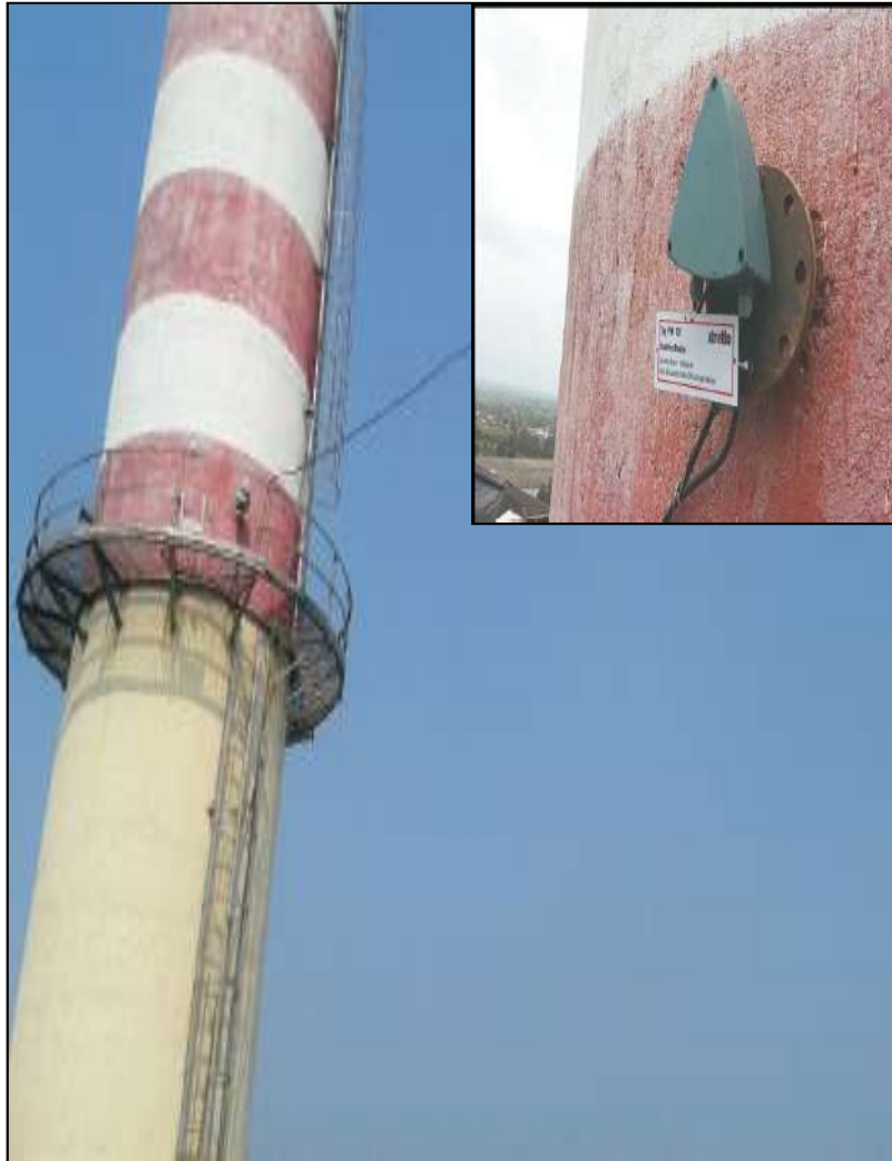
Online Monitoring System
