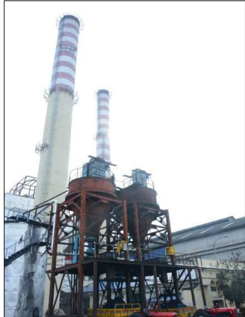
Boiler Ash Handling System
